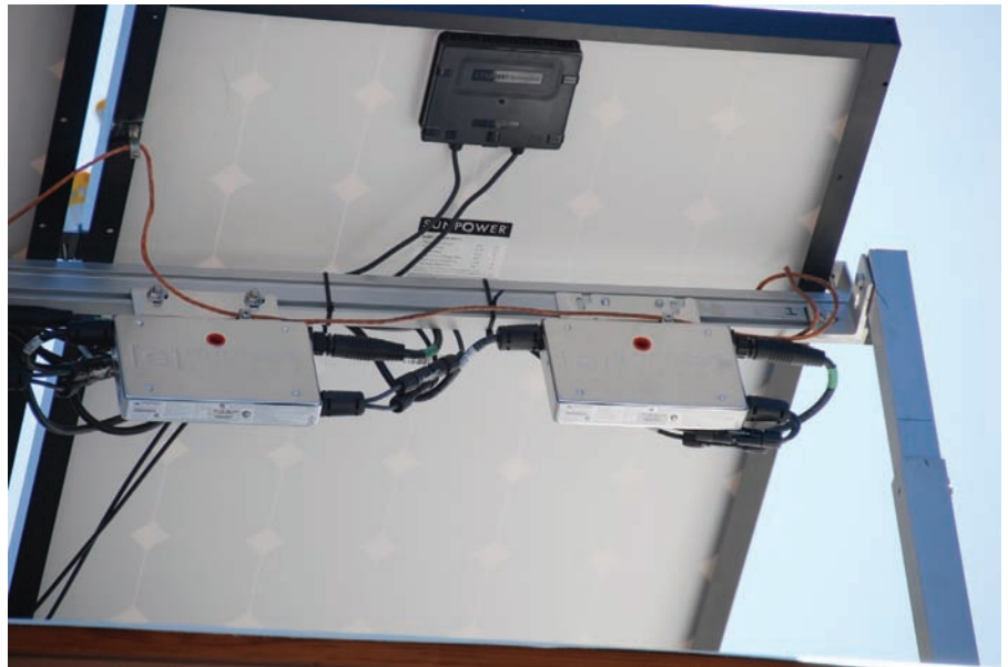
Two Enphase inverters, showing their DC input connections, and AC input and output connections.
