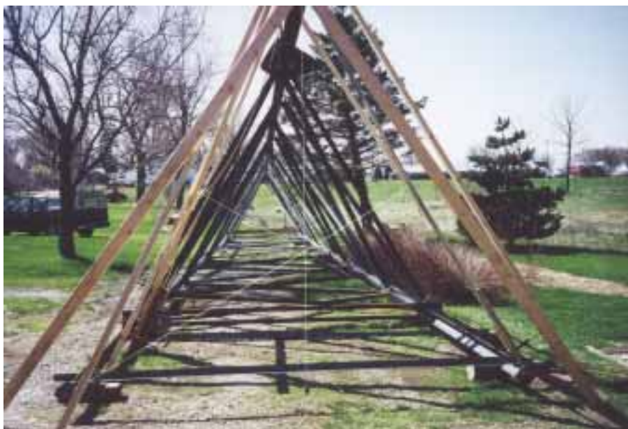
Alignment is crucial for the tower pieces to fit together and to be structurally sound. But a three-legged, tapered tower has no plumb component, so string lines were used to create a center line for reference.
