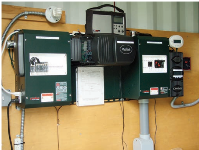
An off-grid system will require batteries and a charge controller, as well as an inverter and disconnects common to all system configurations.
