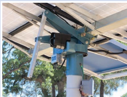
Wattsun tracker gimble and drive system.
