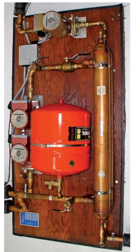
An external, tube-in-shell heat exchanger (far right) with other balance of system components, like circulator pumps (far left) and an expansion tank (center).
